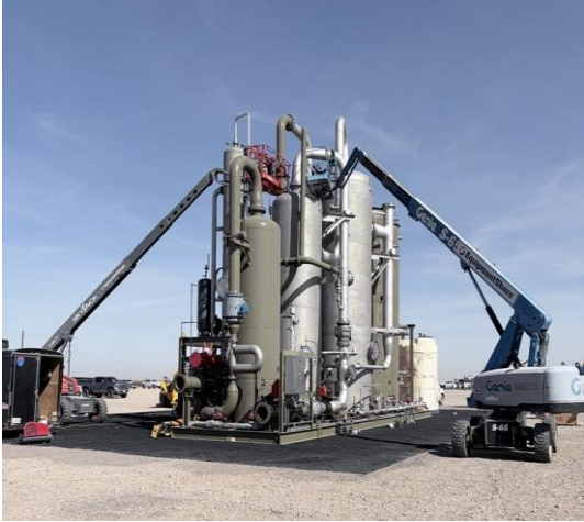
Consolidated Gas Treating Infrastructure
