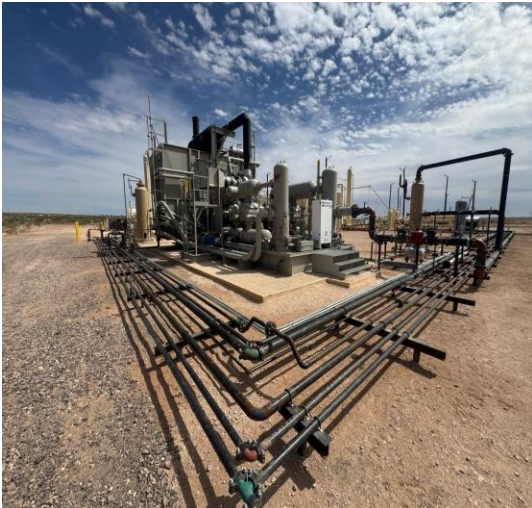
Centralized Compression & Artificial Lift
